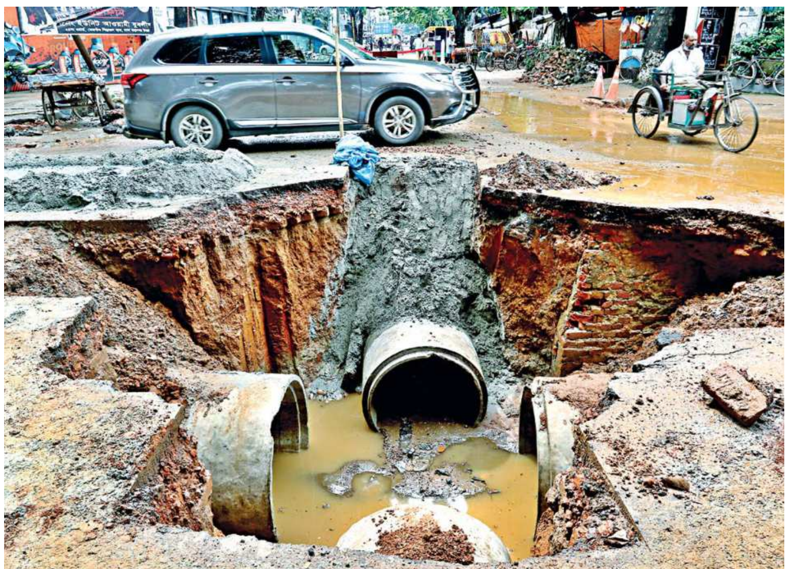
At Tejgaon Industrial Area, a portion of the road near Re-Rolling Mills Bot Tola has been dug up to facilitate DNCC's sewage development works. But with no barricades or tapes in place, the spot carries enormous potential for accidents, which was only made worse by the last few days' rainfall. This photo was taken yesterday.
