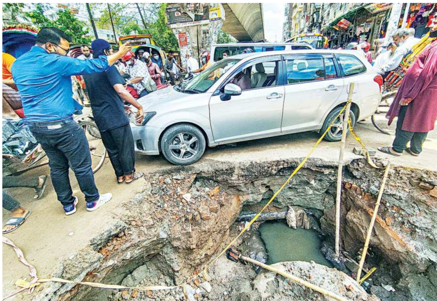
A car struggles to negotiate a road narrowed by a trench dug by the Dhaka South City Corporation for development work in the capital's AHM Kamruzzaman Sarani Banga Bazar. City dwellers have long been suffering due to this situation. The photo was taken yesterday.
