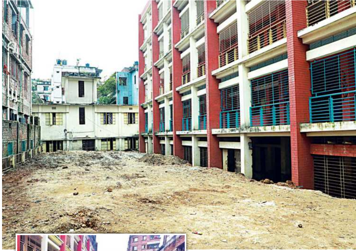
The authorities of Kajalpar Government Primary School in the capital's Jatrabari have solved the institution's waterlogging problem by dumping earth. They made the move after The Daily Star ran a multimedia report on the problem in August. Inset, a previous photo showing how the school premises remained submerged in murky greenish water.
