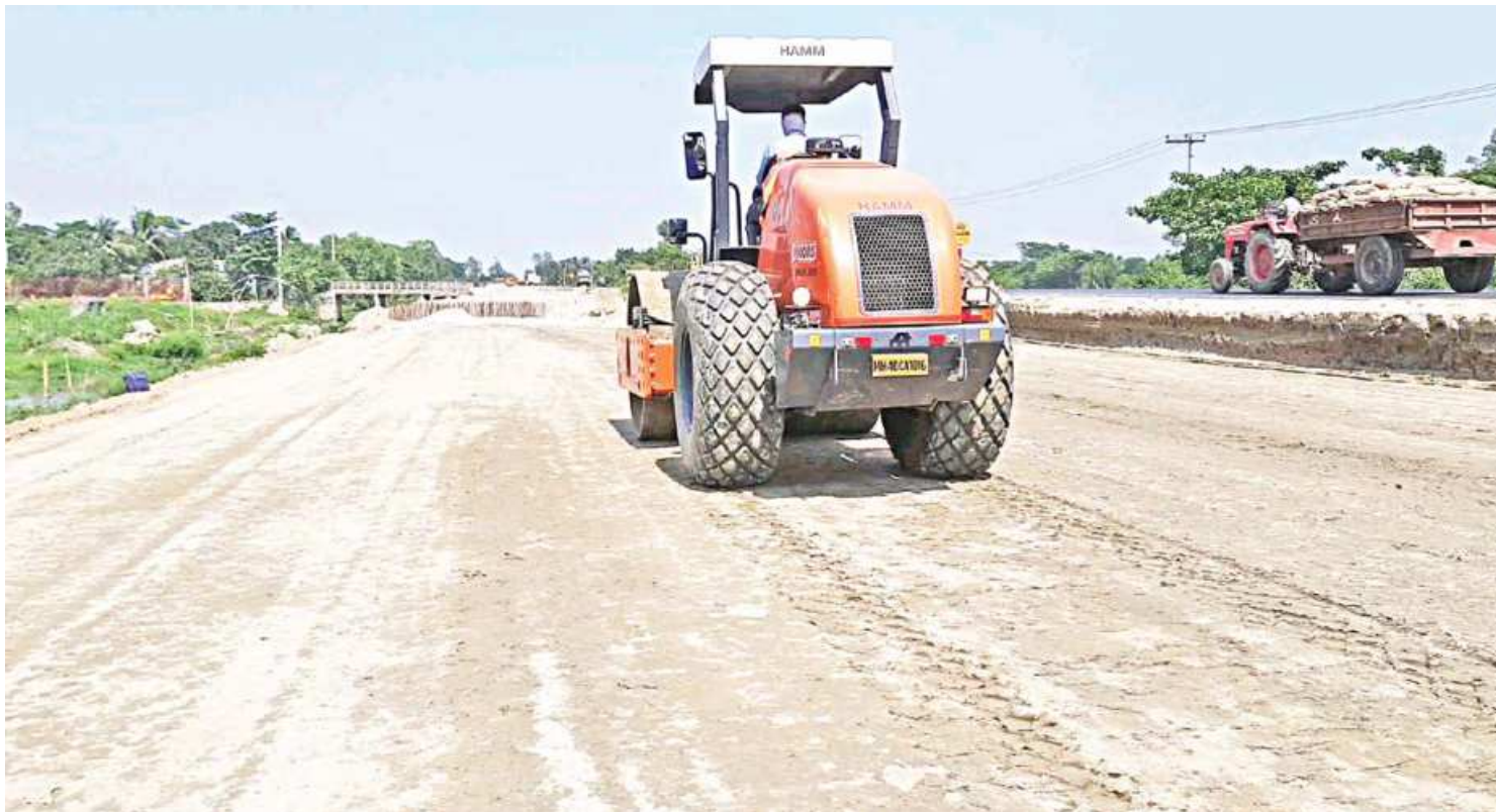
Work has accelerated on a project over widening a 51-kilometre road from the Ashuganj river port to the Akhaura land port to four lanes for smooth transhipment of Indian goods. Scheduled to be completed by 2024, the project will cost Tk 3,567.85 crore, 64 per cent of which is scheduled to come from a second Indian line of credit. The project is expected to establish better communication between Bangladesh and the northeastern part of India, which will ultimately facilitate sub-regional connectivity among South and Southeast Asian countries. The photo was taken yesterday.
