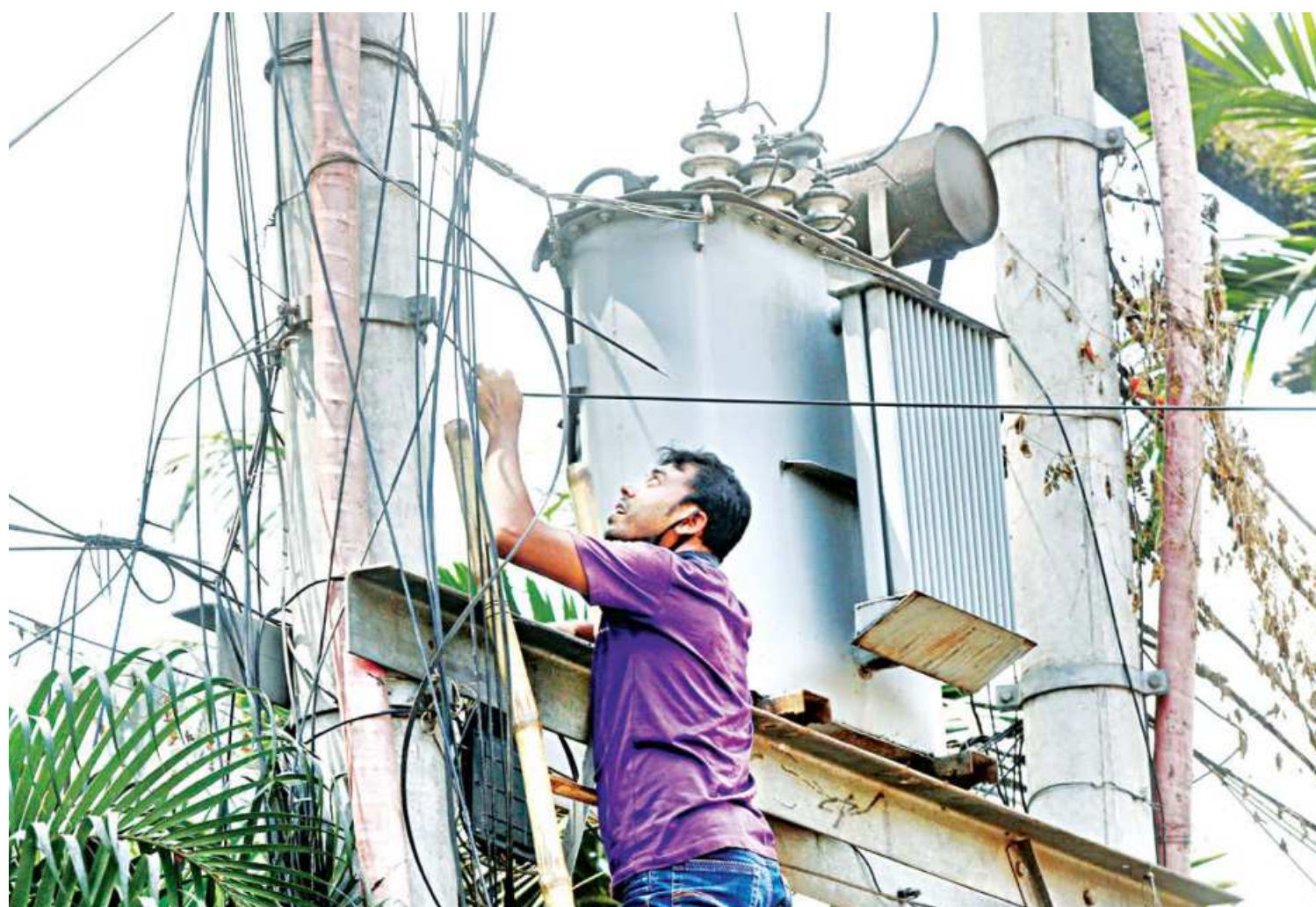
An electrician on a ladder working on repairing an internet cable at the capital's Topkhana Road. He is perilously close to a high-voltage transformer, but he is conducting repairs without taking any visual safety measures such as wearing a safety harness. Such sights are common in the capital and could result in potentially fatal accidents. The photo was taken yesterday.
