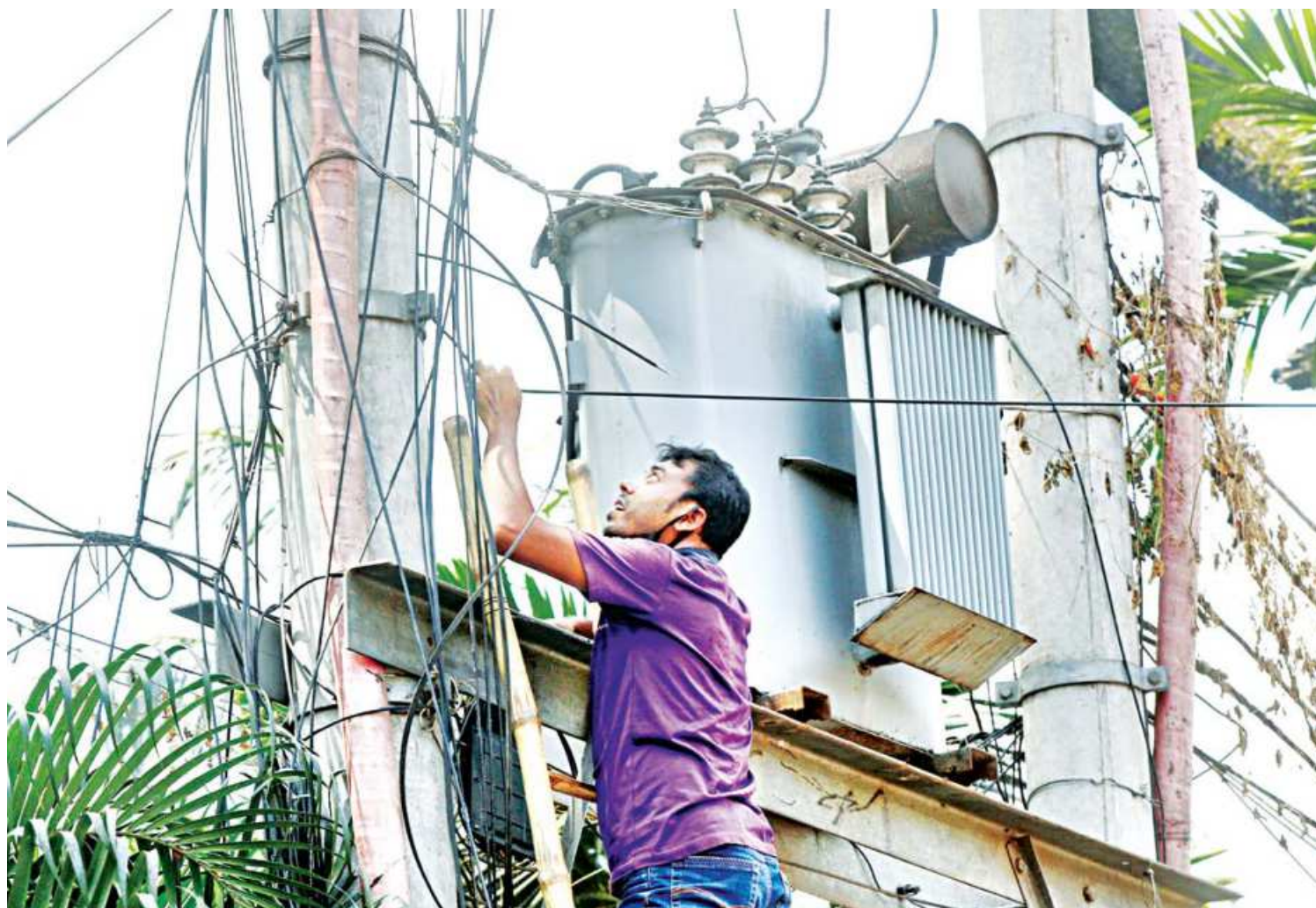
An electrician on a ladder working on repairing an internet cable at the capital's Topkhana Road. He is perilously close to a high-voltage transformer, but he is conducting repairs without taking any visual safety measures such as wearing a safety harness. Such sights are common in the capital and could result in potentially fatal accidents. The photo was taken yesterday.
