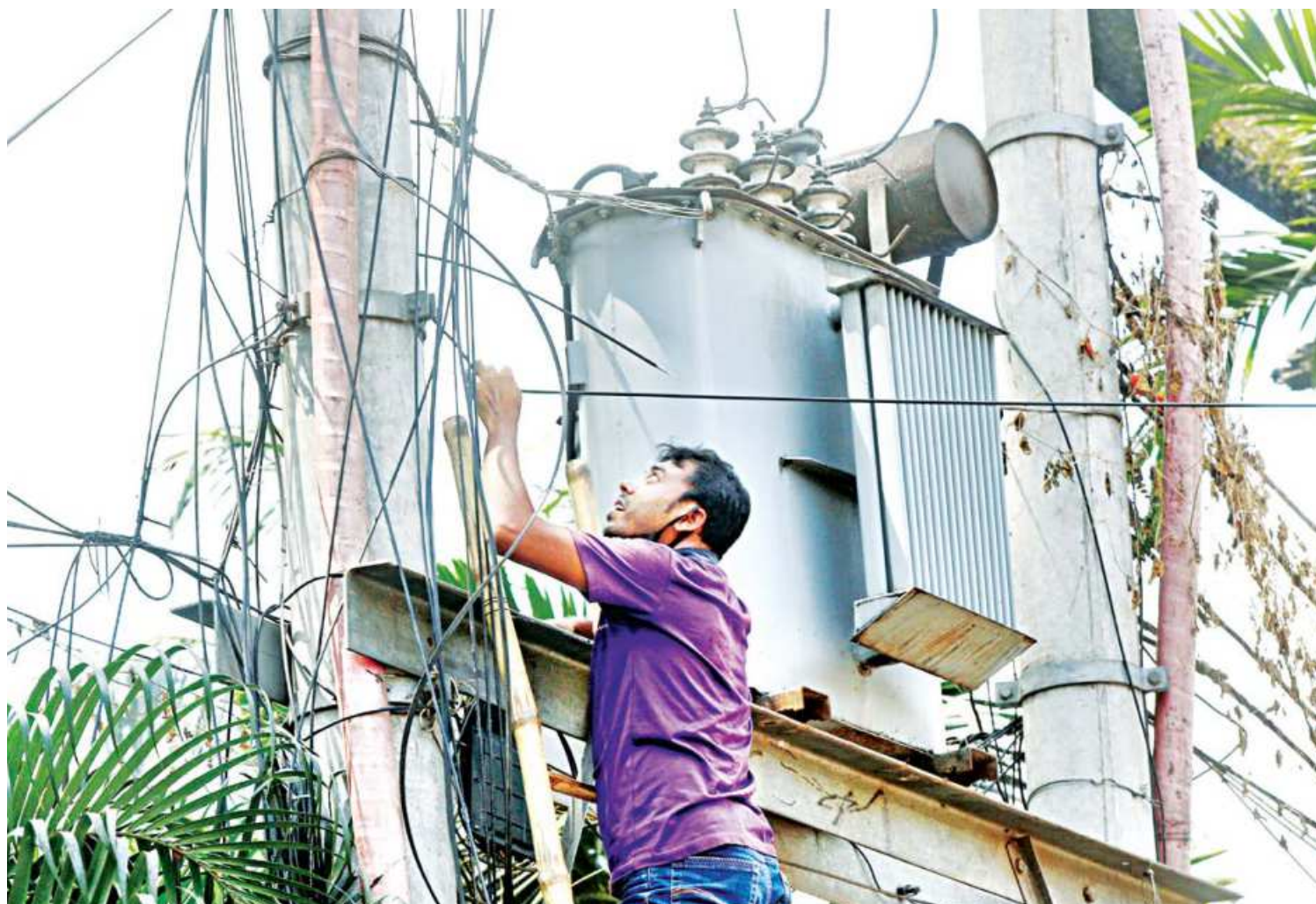
An electrician on a ladder working on repairing an internet cable at the capital's Topkhana Road. He is perilously close to a high-voltage transformer, but he is conducting repairs without taking any visual safety measures such as wearing a safety harness. Such sights are common in the capital and could result in potentially fatal accidents. The photo was taken yesterday.
