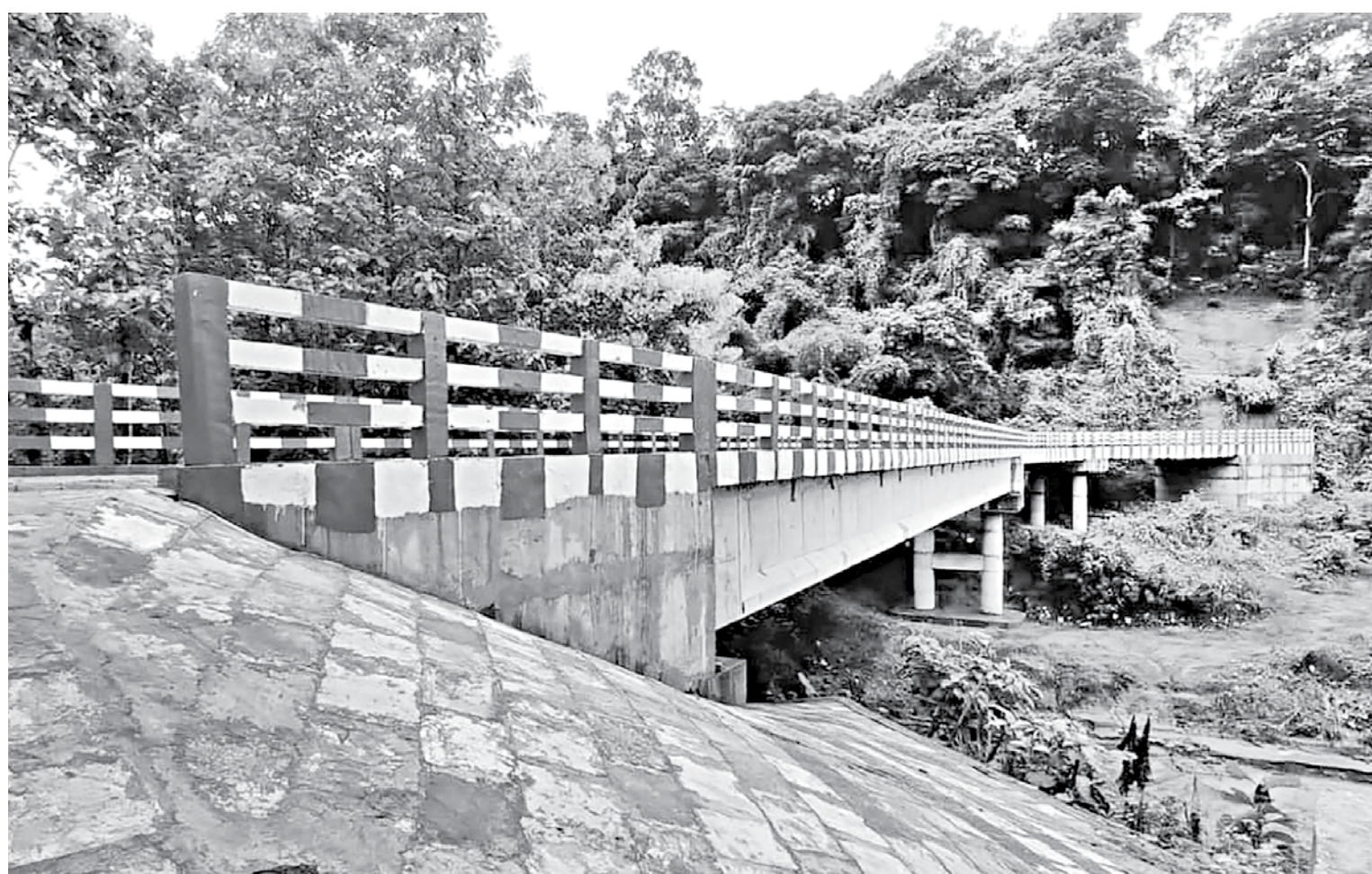
This bridge over Paindu Canal in Bandarban's Ruma upazila lies without any approach roads connected to it
