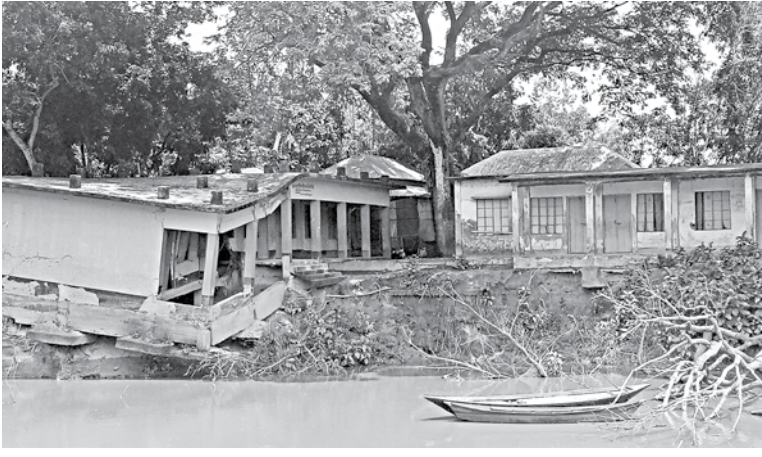
This building of Sarotia Gazi Government Primary School in Tangail's Nagarpur upazila is on the verge of collapse, leaving academic activities of nearly 150 students uncertain. PHOTO: STAR
