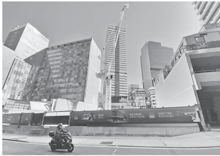
A view of a construction site for a train station on the Sydney Metro, Australia on July 22.
