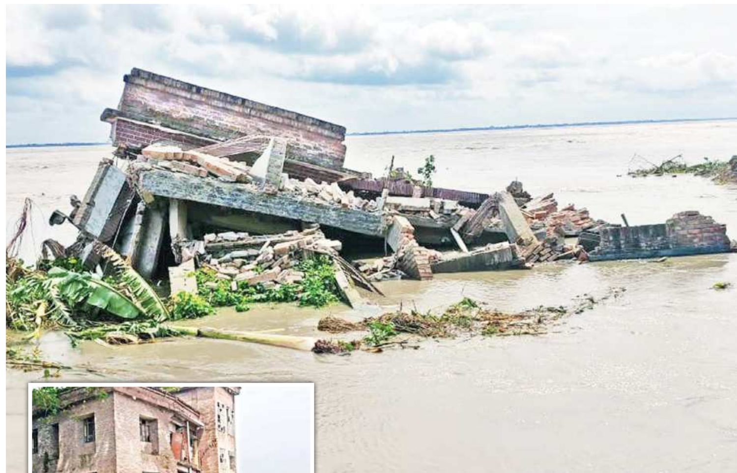
Rubble is what remains after the Azimnagar Union Health and Family Welfare Centre in Harirampur upazila of Manikganj went into the Padma yesterday. Inset, the building being devoured by the river a day before. Story on page 5.
