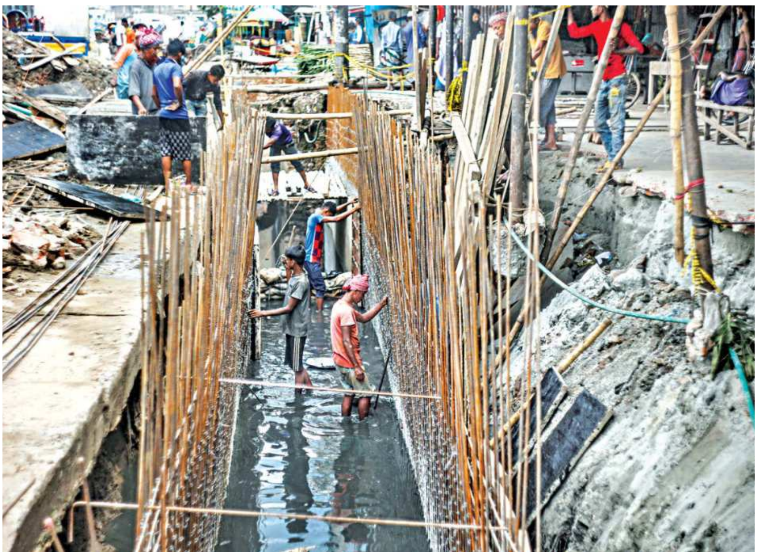
On Jatrabari's Demra Road, DSCC is implementing a project to renovate the area's drainage system to relieve waterlogging issues. But for such a risky undertaking, its workers were not seen wearing any kind of safety gears, with no other protective measures in place either. This photo was taken yesterday.
