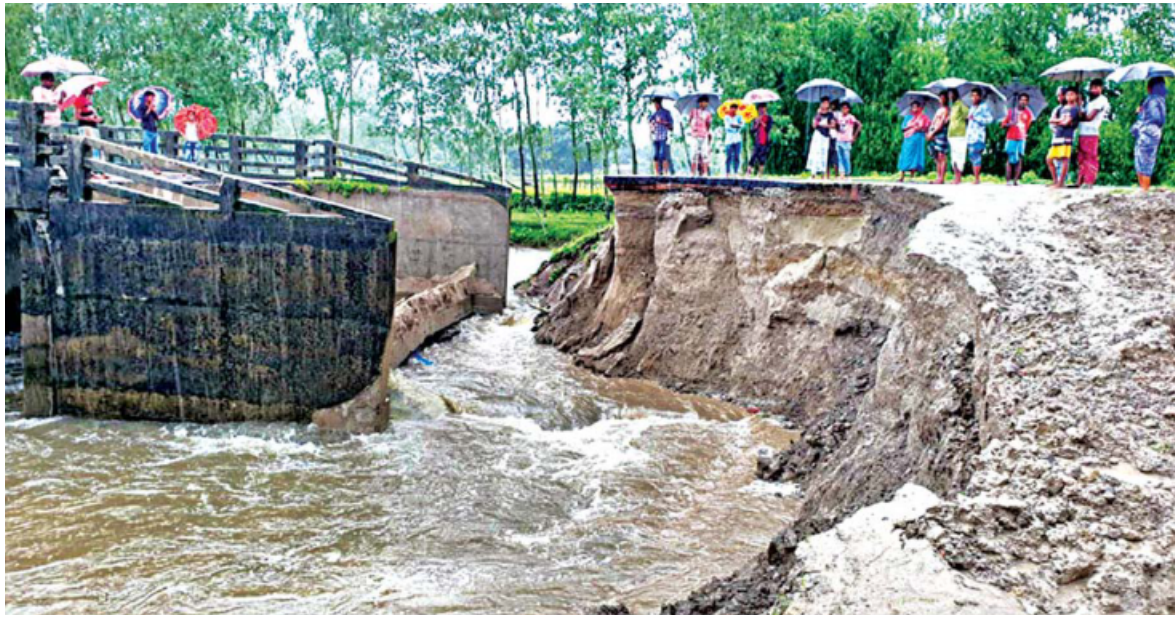
Locals stand on the edge of a collapsed road that led to a bridge on the Panchagarh-Debiganj road in Thakurgaon. Strong currents and rising water levels caused by a flash flood resulted in the collapse of the structures, cutting off road communication. The photo was taken yesterday. PHOTO: QUAMRUL ISLAM RUBAIYAT
