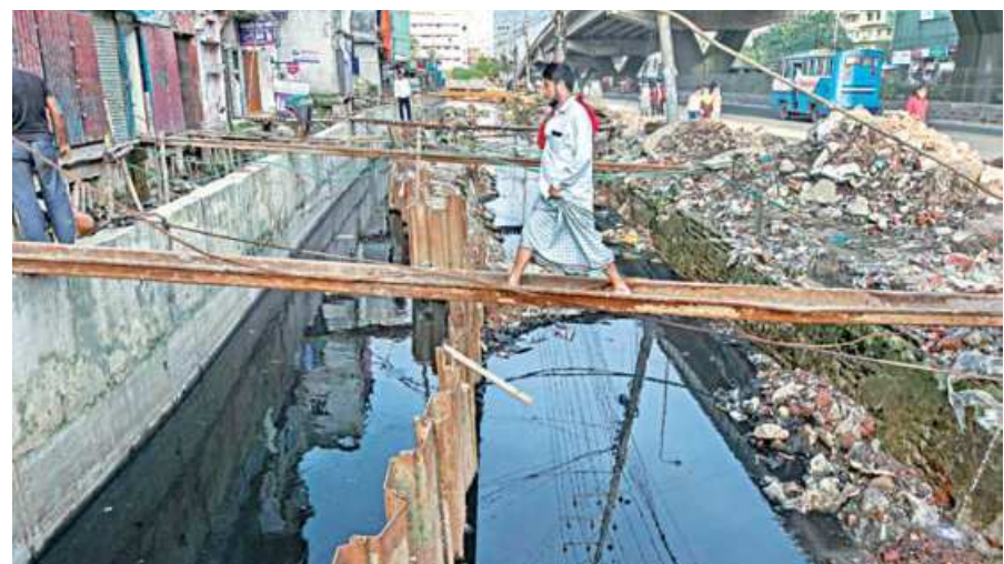
No coverings, no barriers, no warnings, these wider drains of the port city are possible death traps for unsuspecting pedestrians. And when the streets are submerged due to waterlogging, there is no way of knowing where danger lurks. This photo was taken yesterday from Muradnagar area.
