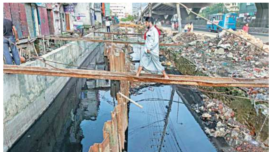
No coverings, no barriers, no warnings, these wider drains of the port city are possible death traps for unsuspecting pedestrians. And when the streets are submerged due to waterlogging, there is no way of knowing where danger lurks. This photo was taken yesterday from Muradnagar area.
