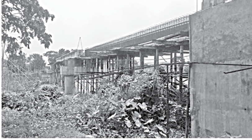
Though set to be completed by March 2020, the planned 75-metre bridge over Bangshi river only has 40-metre of work done as of date.
