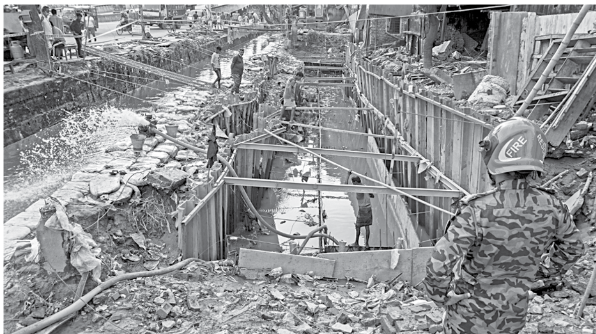
Even after a whole day of rescue attempts, firefighters could not find vegetable trader Saleh Ahmed, who fell into a canal at port city's Muradpur area on Wednesday. Workers were siphoning water out of the canal using hoses till 5pm yesterday, in hopes of spotting the man.
