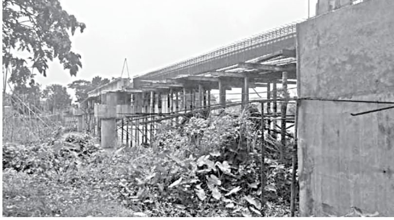
Though set to be completed by March 2020, the planned 75-metre bridge over Bangshi river only has 40-metre of work done as of date. PHOTO: STAR
