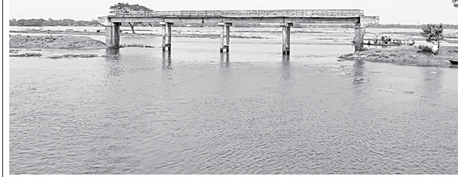
Signs of decay are visible all over the bridge -- on Nayakhal canal in Dharkhar union of Brahmanbaria's Akhaura upazila -- that was neither open nor got any approach road in the last 22 years. Several of its pillars are already damaged and parts of its guard rails are missing. The photo was taken recently.
