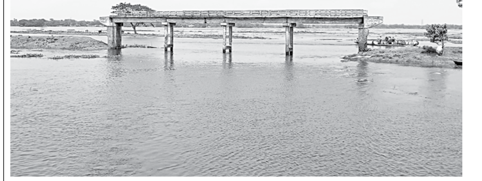
Signs of decay are visible all over the bridge -- on Nayakhal canal in Dharkhar union of Brahmanbaria's Akhaura upazila -- that was neither open nor got any approach road in the last 22 years. Several of its pillars are already damaged and parts of its guard rails are missing. The photo was taken recently.
