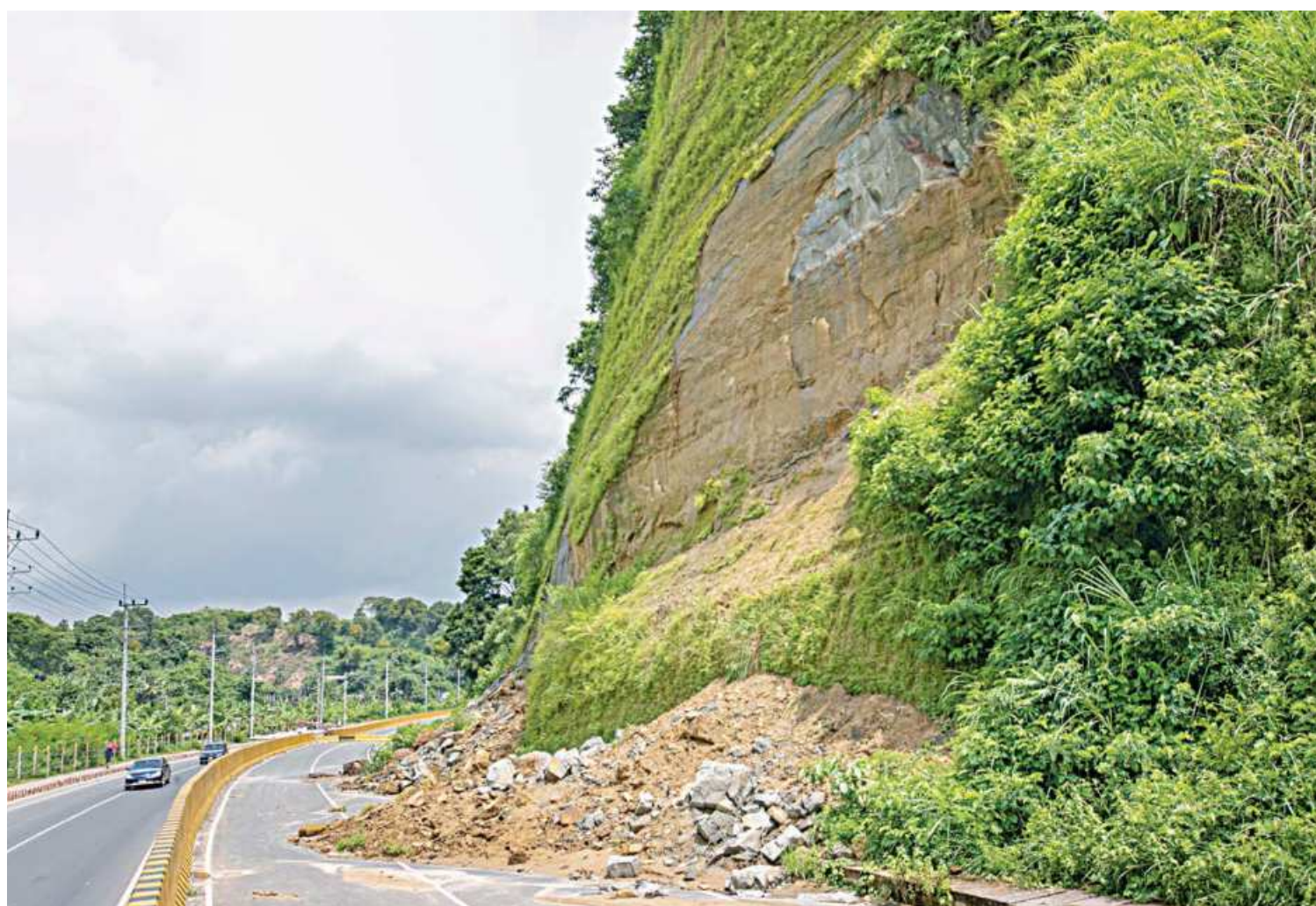
This dual-carriageway, connecting Foudjarhat and Bayezid in Chattogram, was built cutting part of a hill. A large chunk of earth recently fell on the road and the authorities, deeming it unsafe, have closed off one side of the road at Jangal-Salimpur and set up contraflow on the other side. The photo was taken yesterday.
