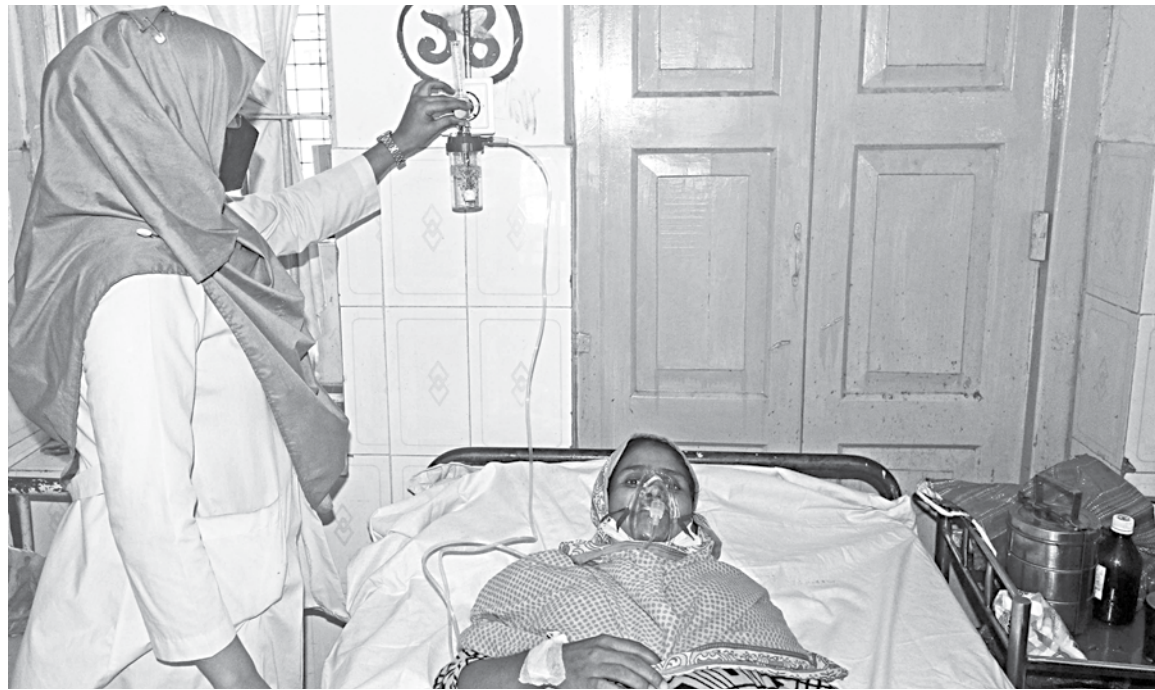
Oxygen is being administered to a Covid patient from a newly installed outlet of the centralised oxygen supply system at Birganj Upazila Health Complex. The photo was taken recently. PHOTO: KONGKON KARMAKER
