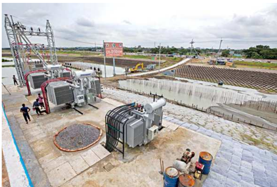
Construction work for Bay Terminal, a long-awaited mega expansion project of the Chattogram port, has gained momentum as the government has set 2024 to start operation of the terminal. The photos were taken yesterday.
