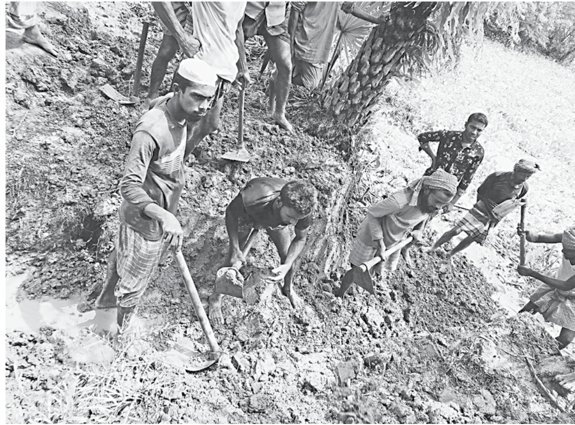
Villagers, at the directive of local public representatives, removing one of the five illegal dams that were built ten years ago in Kaunia canal under Amtali upazila of Barguna. The Photo was taken on August 13.
