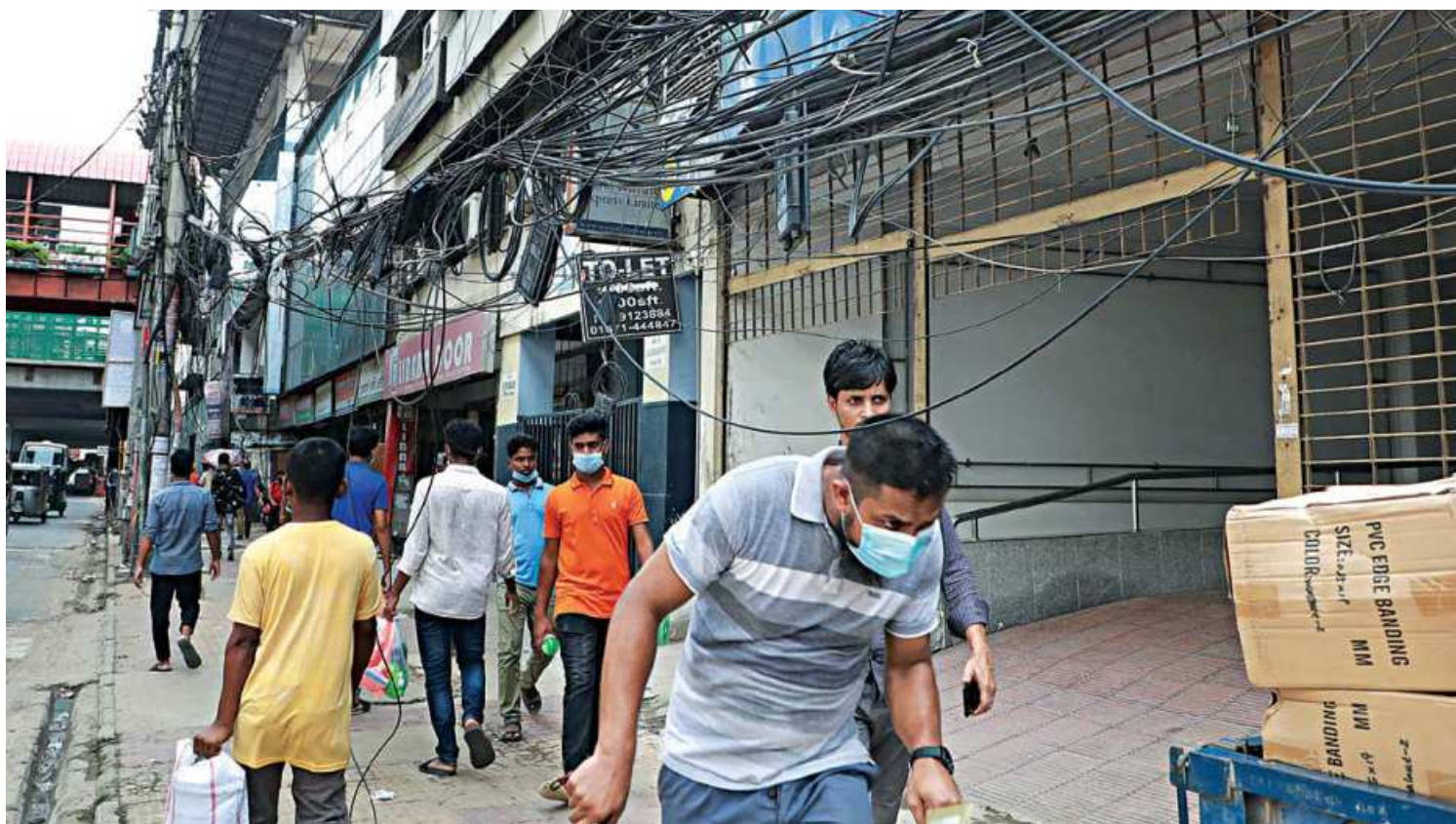
AN OBSTACLE COURSE NO ONE ASKED FOR... Dangling electric, telephone, and internet cables have been around for so long that citizens have become desensitised to them. But ever so often, one will come off the entanglement and hang low, causing a significant but barely noticed hassle for commuters passing by, along with the electrocution risk that comes with it. On top of this, other obstacles on footpaths, like the loaded pickup-van pictured on the right, cause additional difficulty for pedestrians. This photo was taken from the capital's Kazi Nazrul Avenue near Karwan Bazar yesterday.
