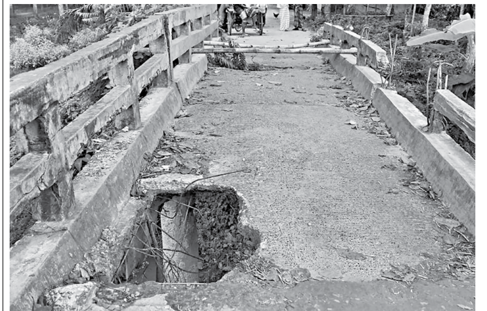
People cross this damaged bridge over Charakhali Canal at Fukurhati village in Faridpur's Bhanga upazila amid risk of accidents.
