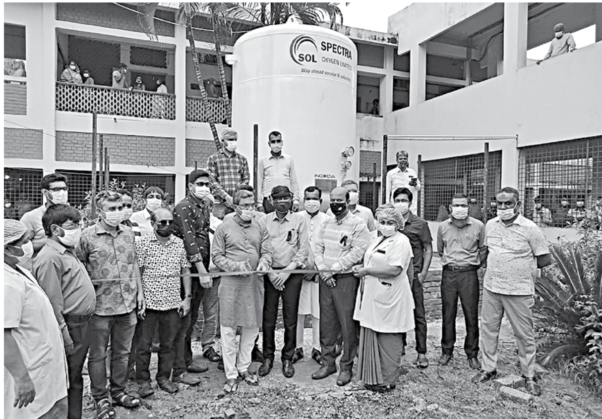
A central oxygen supply plant was inaugurated at 250-bed Pabna General Hospital on August 7. Pabna-5 constituency lawmaker Golam Faruk Khandakar Prince formally launched the service on the hospital premises.
