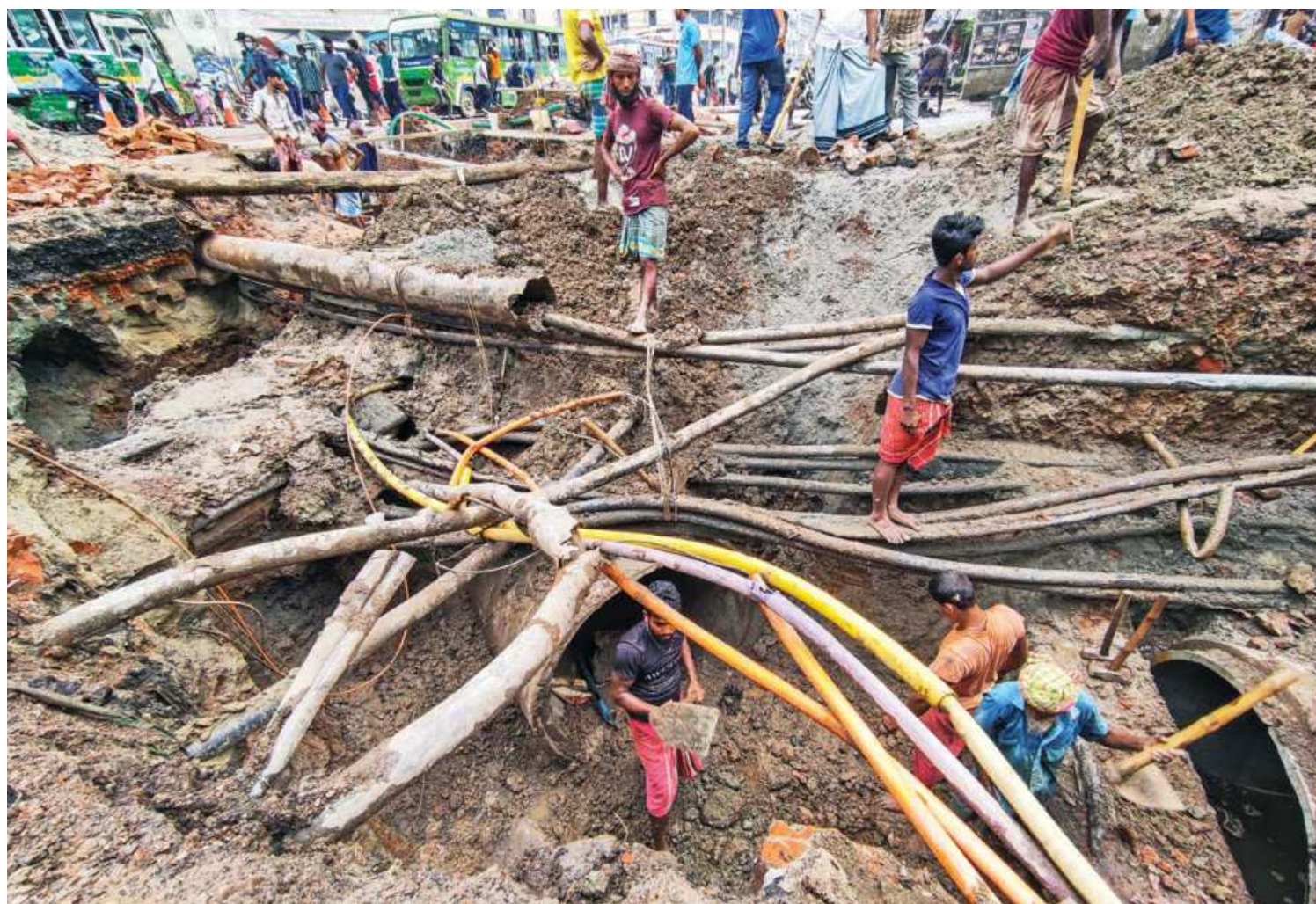
Risks of serious accidents do not seem to be on its mind as Dhaka South City Corporation continues its work on the development of the sewage system below Hanif flyover in Gulistan's Phulbaria without taking enough safety measures. The photo was taken yesterday.
