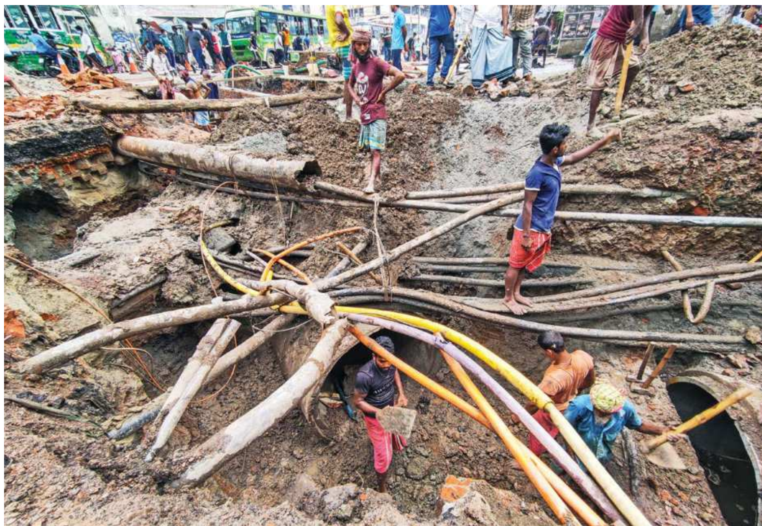
Risks of serious accidents do not seem to be on its mind as Dhaka South City Corporation continues its work on the development of the sewage system below Hanif flyover in Gুলিস্তান's Phulbaria without taking enough safety measures. The photo was taken yesterday.
