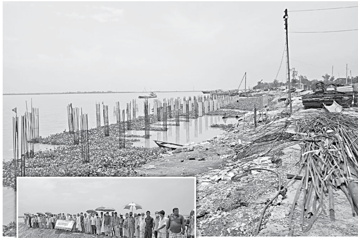
The construction site of the modern river port in Pabna's Nagarbari under Bera upazila. Inset, affected landowners in a human chain demand compensation for the land acquired from them. The photo was taken recently.
