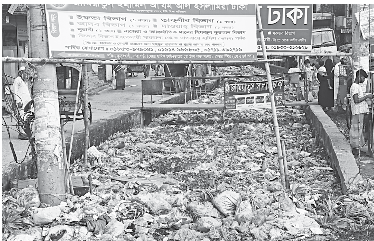
Once part of Jatrabari's Kutubkhali canal, this waterbody has been turned effectively into a large gutter due to construction work around it and then filled up with waste to the point no water passes through it. Only a few months ago, Dhaka South City Corporation had cleaned it up, but that effort has gone down the proverbial drain, judging by the looks of it. The photo was taken yesterday.
