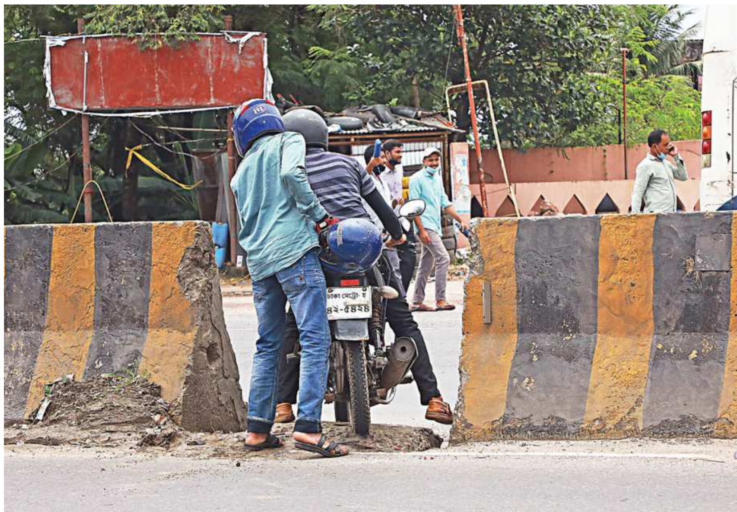
A motorbiker attempts to cross over from one side of Chittagong Road illegally through a broken part of the road divider, while his pillion gets off the bike and helps him. On a wide road where vehicles often ply at high speed, such attempts can be very dangerous. The photo was taken near Matuail yesterday.
