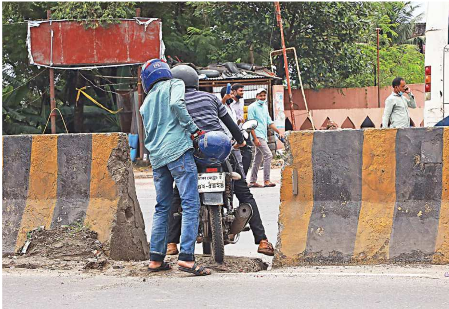
A motorbiker attempts to cross over from one side of Chittagong Road illegally through a broken part of the road divider, while his pillion gets off the bike and helps him. On a wide road where vehicles often ply at high speed, such attempts can be very dangerous. The photo was taken near Matuail yesterday.
