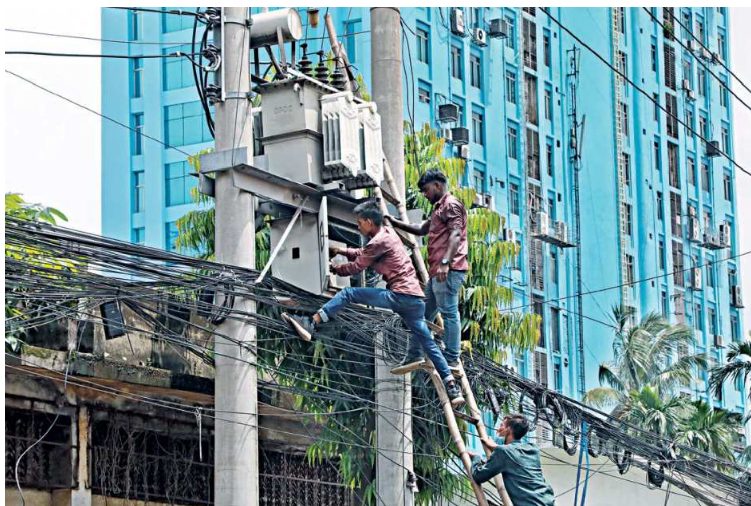
With one foot on the ladder and the other resting precariously on wires, an electrician along with his workmates is busy working on a transformer. One misstep at any point of the work may lead to a serious accident. This photo was taken yesterday from the capital's Tejjanga.
