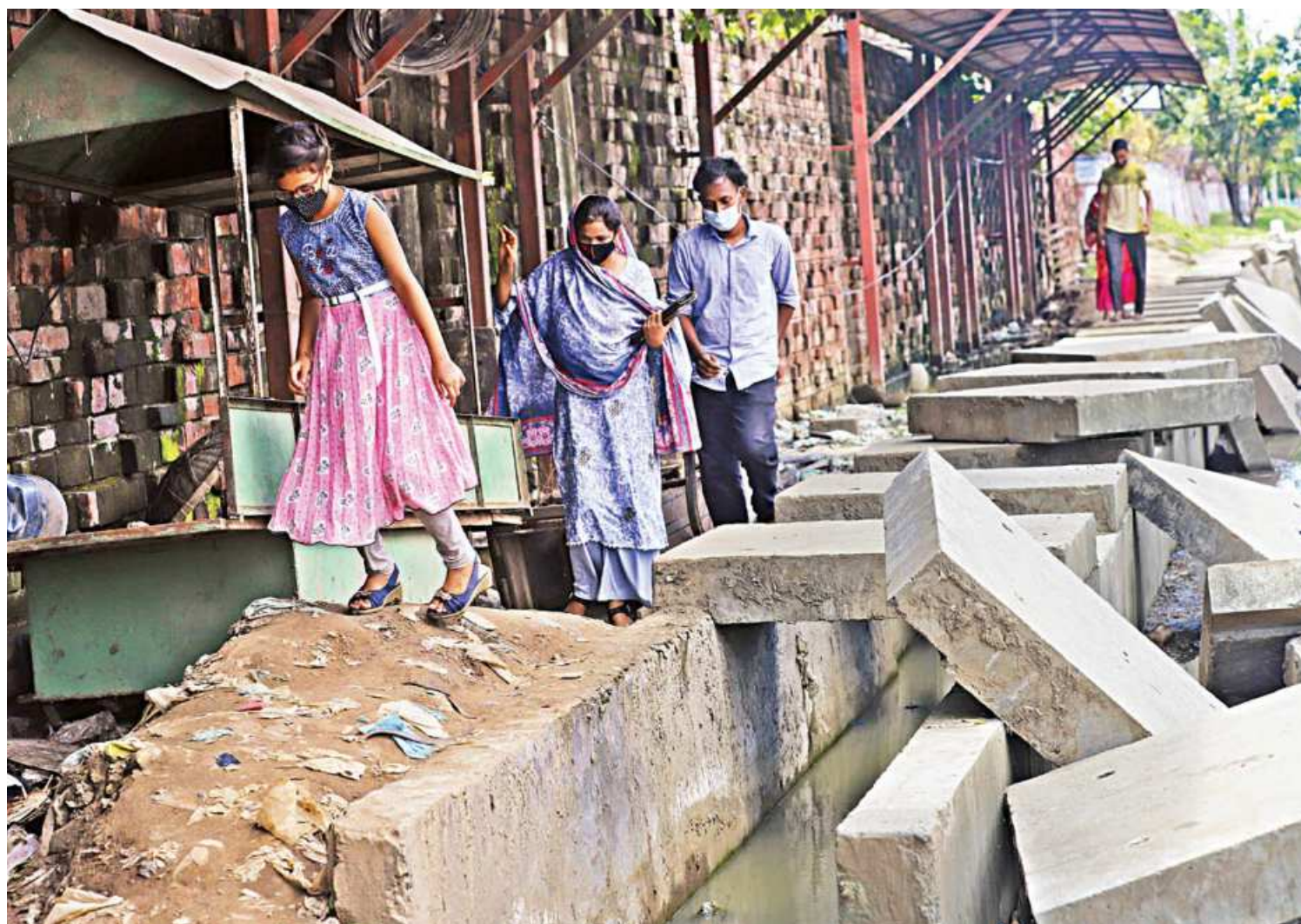
People struggle to walk by a broken footpath, which has not been repaired for over a year now, near the airport road roundabout. The photo was taken yesterday.
