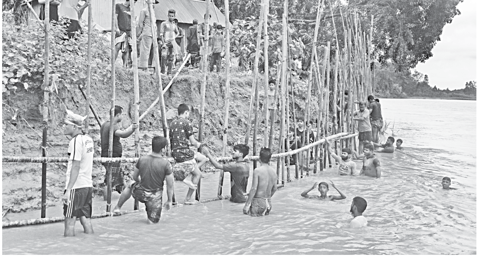
Locals join voluntary service to construct an embankment on Louhajang river to save an Eid congregation ground, a graveyard and a dakhil madrasa from erosion.
