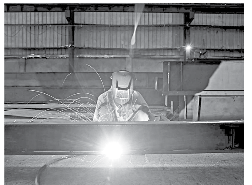
A labourer welds an iron pillar at a building material factory in an industrial area in Dasna, in the central Indian state of Uttar Pradesh, India.
