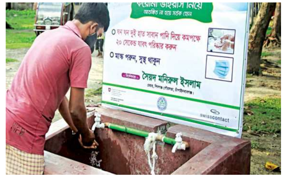
Eight handwashing basins are installed at a mango market in Chapainawabganj.
