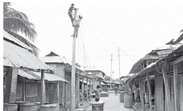
Isolated Rangabali upazila of Patuakhali to get much-anticipated electricity connection by August 15.
