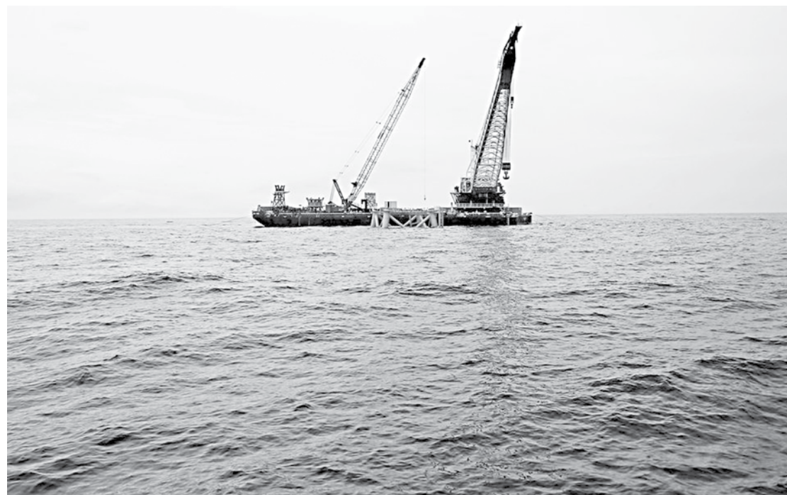
A crane hangs over the first jacket support structure installed to support a turbine for a wind farm in the waters of the Atlantic Ocean off Block Island, Rhode Island.
