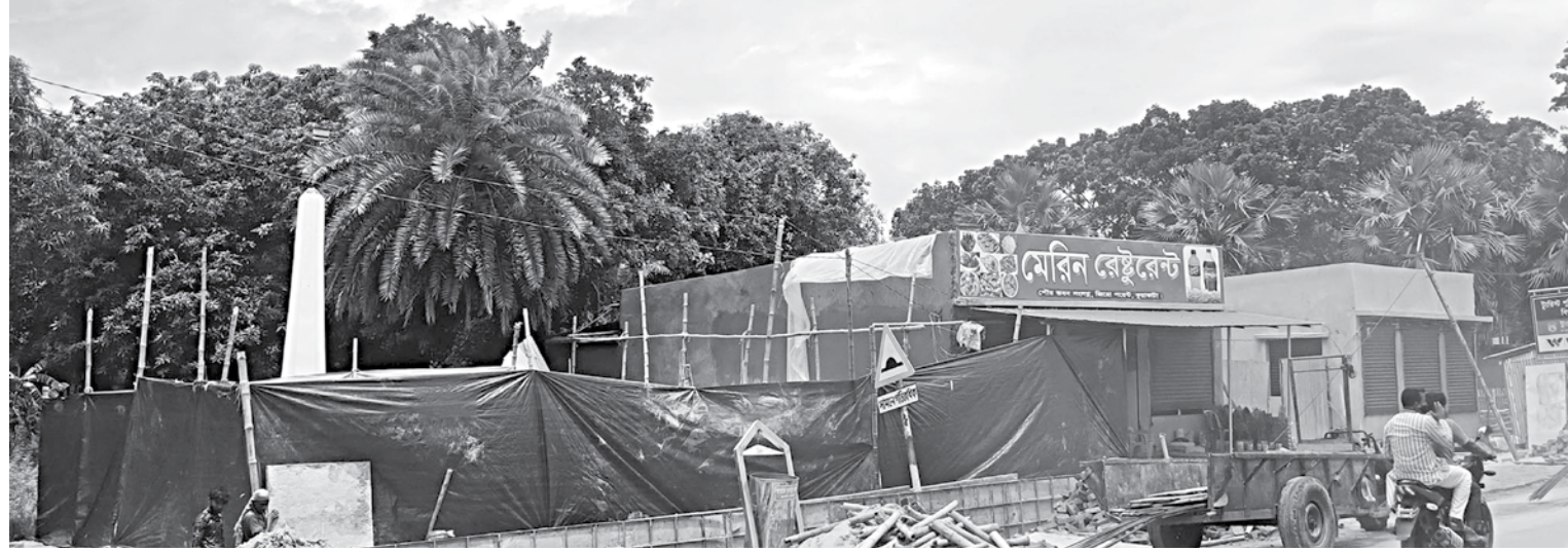
Concealed behind polythene sheets, construction of shops is underway on Patuakhali-Kuakata highway near Kuakata Municipality building. The structures under construction and the ones already built are on the land that belongs to a two hundred year-old Buddhist temple (visible behind the polythene covering), monastery and graveyard of Rakhine community.
