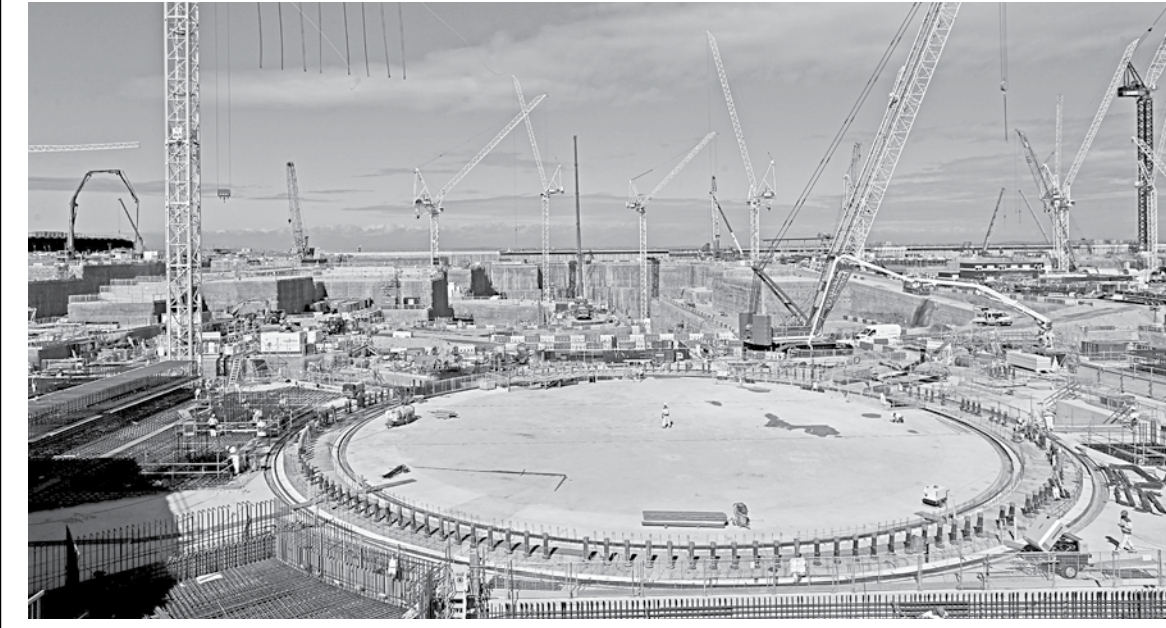
Construction takes place at the Hinkley Point C nuclear power station site, near Bridgwater, UK. REUTERS/FILE
