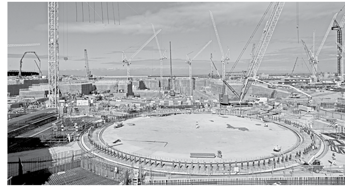
Construction takes place at the Hinkley Point C nuclear power station site, near Bridgwater, UK.
