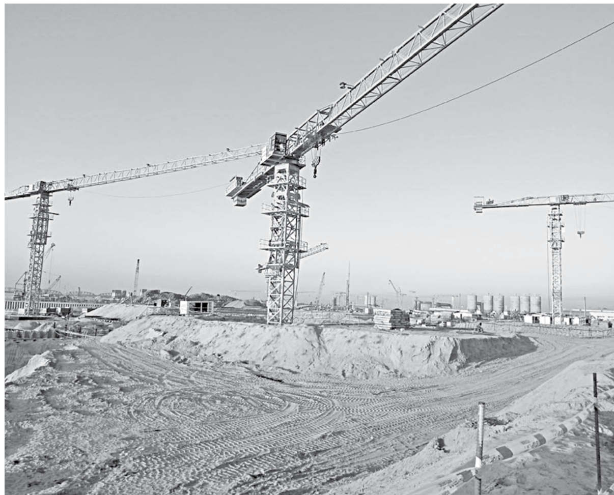
Construction work of Rooppur Nuclear Power Plant Project, the country's first nuclear power plant, is going on in full swing and expected to be completed within the schedule time.
