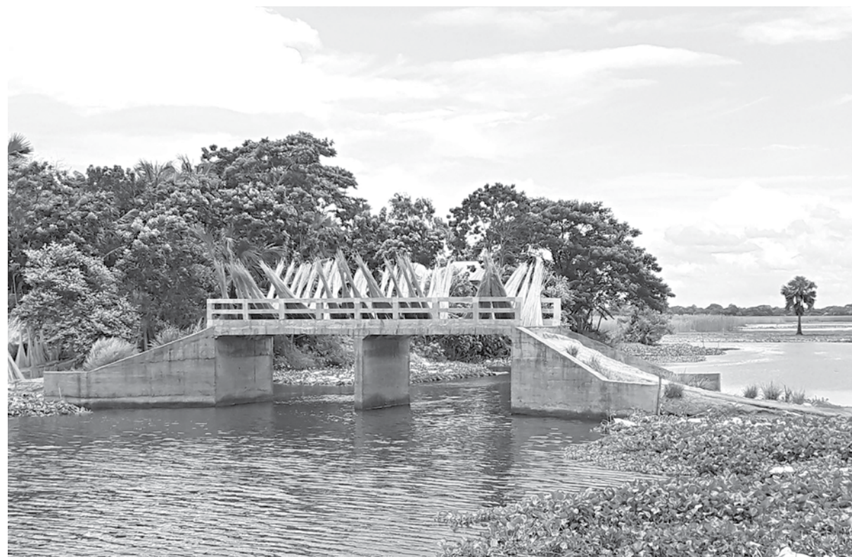
This bridge, built over Bedakhali canal at Tugholdia village in Faridpur's Saltha upazila nearly two years ago, lies unusable due to lack of approach roads on both sides. Ministry of Relief and Disaster Management built the 40-foot long bridge in 2018-2019 fiscal year spending over Tk 31 lakh.
