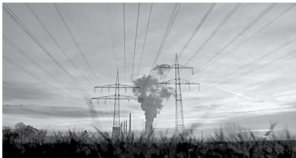
General view of electricity pylons and power lines leading from the Uniper coal power plant in Hanau, Germany.
