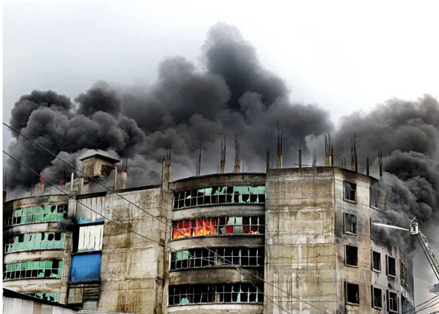
Smoke billows from the six-storey factory building of Hashem Foods as firefighters try to put out the flames yesterday, hours after a fire broke out at the factory in Karnagop area of Narayanganj's Rugganj upazila. The massive blaze swept through the building, leaving at least 52 people dead. More photos on page 3.
