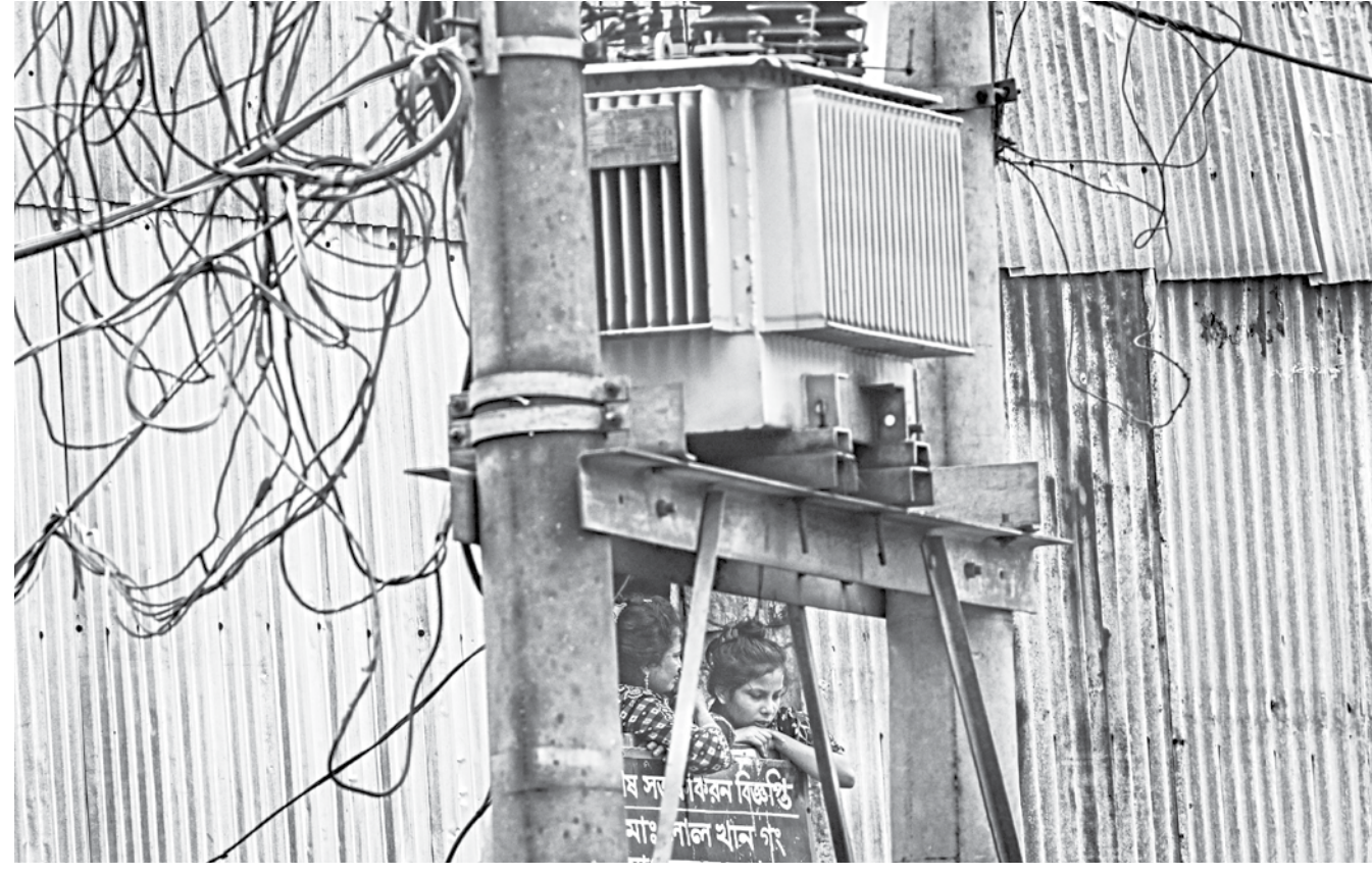
A week after the accident at Lalbagh's Islambagh that killed two people, electricity transformers in the area still sit dangerously close to residential establishments. This photo was taken yesterday.
