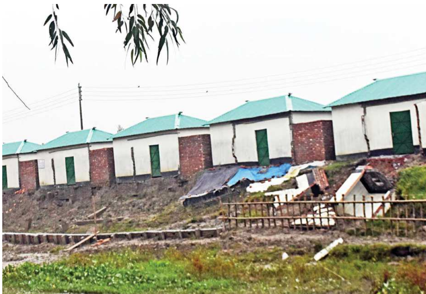
Seven houses built for homeless people in Koyerkhali area of Bogura's Sherpur upazila under the Ashrayan-2 project have partially collapsed following moderate rainfall four days ago. Locals blamed poor quality construction work. The photo was taken on Tuesday.
