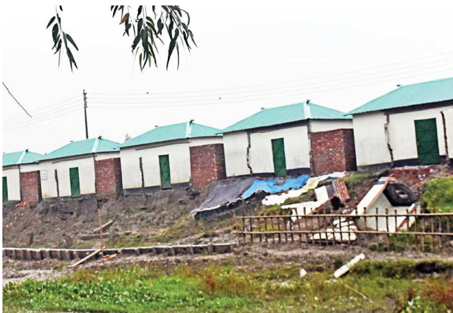
Seven houses built for homeless people in Koyerkhali area of Bogura's Sherpur upazila under the Ashroyon Project-2 have partially collapsed following moderate rainfall four days ago. Locals blamed poor quality construction work. The photo was taken on Tuesday.
