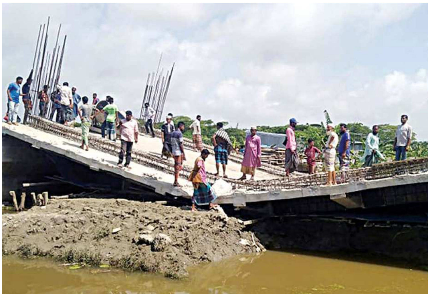
An under-construction bridge collapsed in Kuakata municipality's Dobhashipara area on Sunday. Locals claim the accident occurred due to a design error and incomplete piling. They also alleged that the organisation concerned in building the bridge is a fraud.
